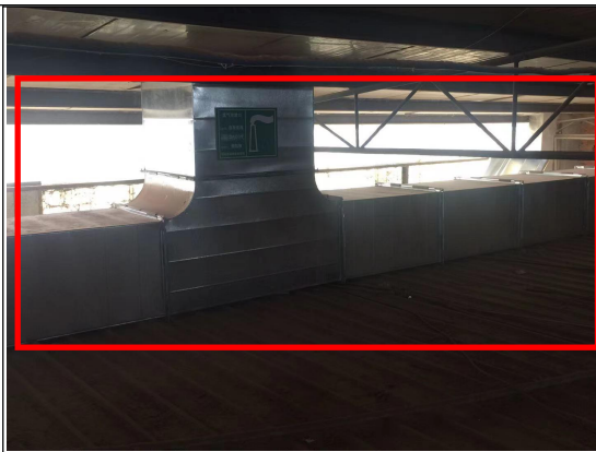
1#车间灰工粉尘废气排气筒1#
